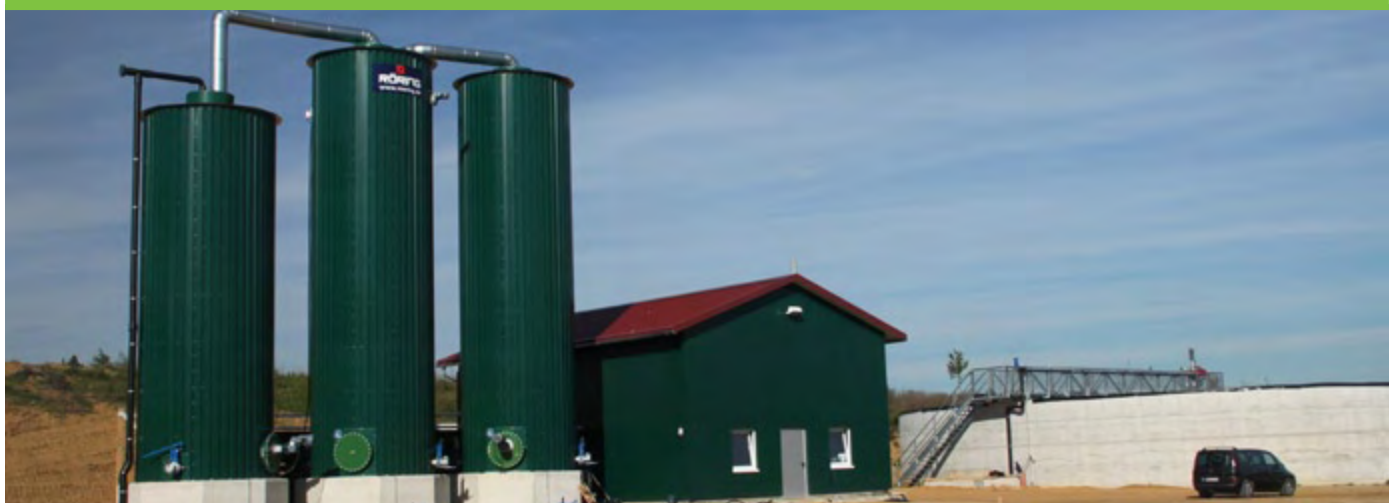
UDR-fermenters and reflow tank from manufacturer Roering GmbH with diameters of 3 meters and heights of 9 and 11 meters.
