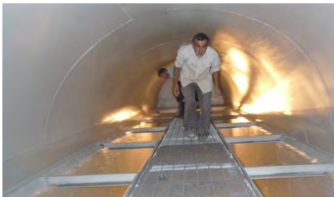
Waste water separation vessel
