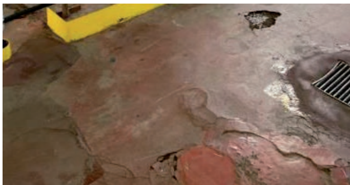
The damaged floor prior to renovation
