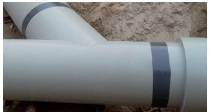
After assembly the welding seams were additionally coated on site with a protective layer
