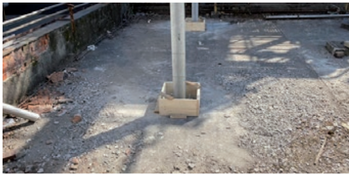
The damaged concrete before renovation.
